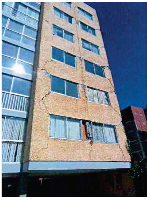
Figure 10-15 Damage to west façade masonry walls (Dirac Ingenieros Consultores, 2019b).
