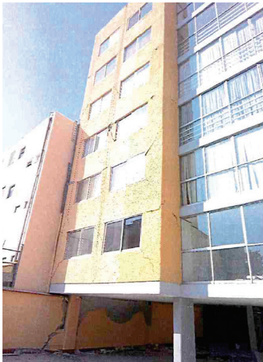
Figure 10-18 Photograph showing damage to first story masonry walls and close proximity of adjacent building in south boundary (Dirac Ingenieros Consultores, 2019b).
