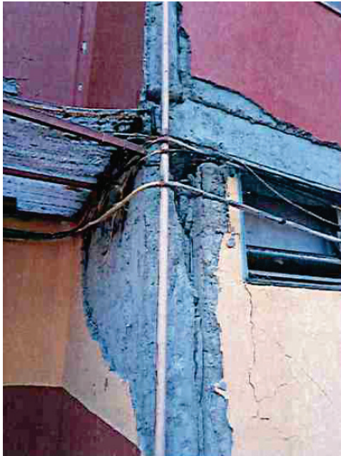
Figure 10-14 Damage at the edge of first story structural wall (Dirac Ingenieros Consultores, 2019b).
