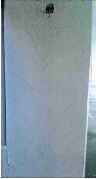
Figure 10-13 Inclined cracks observed in first story column (Dirac Ingenieros Consultores, 2019b).
