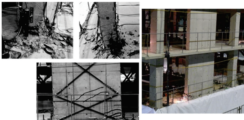
Figure 4-9 Observed damage in first story of shear walls (adapted from Nagae et al., 2015). Top left photos: base of wall at Gridline C closer to Gridline 2 (left) and Gridline 1 (right); Bottom left photo wall base at Gridline A; Photo on the right shows wall at Gridline C.
