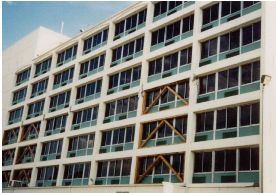
Figure 7-12 Structural damage to columns of south exterior frame after 1994 Northridge Earthquake (Concrete Coalition, 2019). Braced frames added after the earthquake as temporary lateral support.
