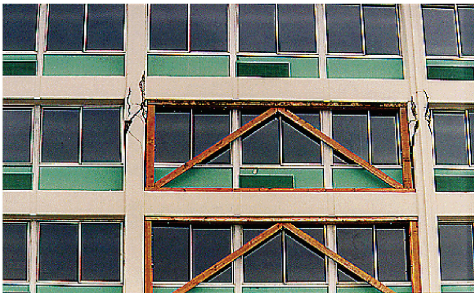
Figure 7-13 Structural damage to fifth floor columns of south exterior frame after 1994 Northridge Earthquake (Naeim et al., 2005). Braced frames added after the earthquake as temporary lateral support.
