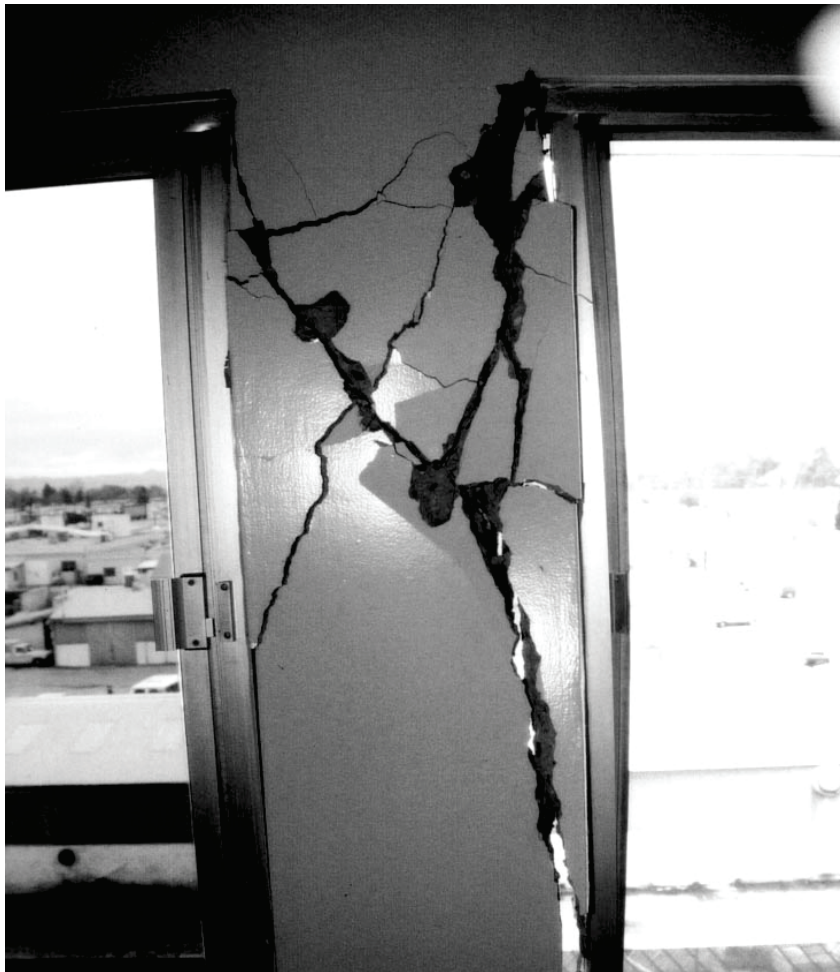
Figure 7-17 Shear distress in Column A5, fifth floor (Trifunac et al., 1999).
