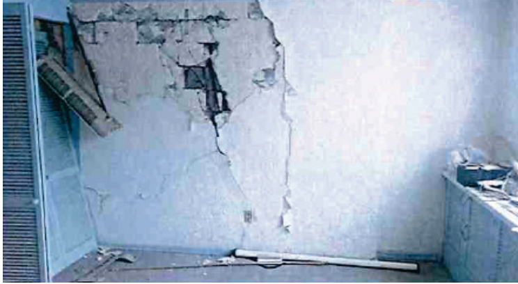
Figure 10-19 Damage to interior masonry walls in apartment unit (Dirac Ingenieros Consultores, 2019b).
