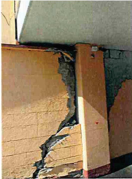
Figure 10-17 Damage to first story masonry walls in north building boundary (Dirac Ingenieros Consultores, 2019b).
