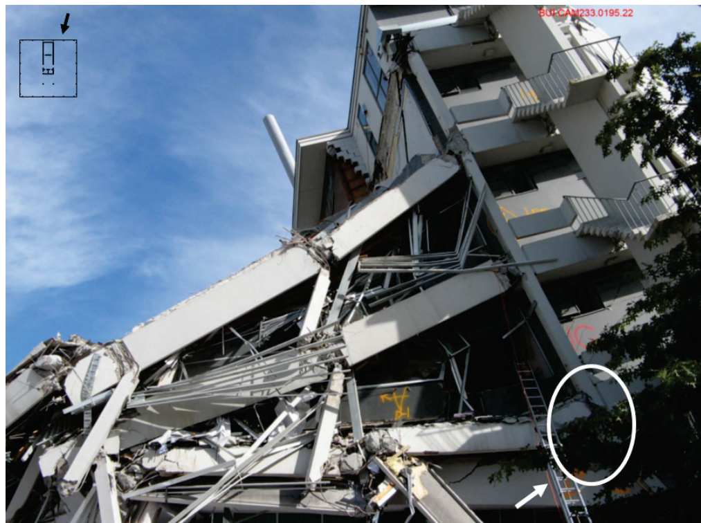
Figure 8-11 Photo showing overview of collapsed building from north; circle indicates location of axial failure of east wall (obscured; adapted from Jury and Sharpe [2011]).
