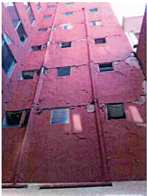
Figure 10-16 Damage to façade masonry walls in north illumination shaft (Dirac Ingenieros Consultores, 2019b).
