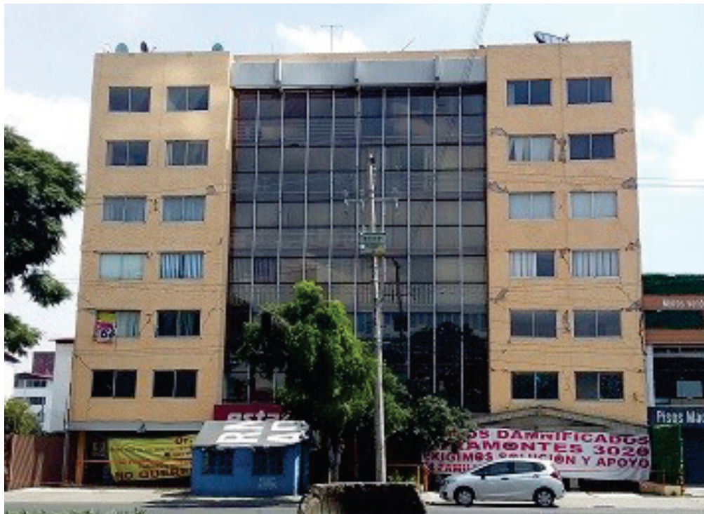
Figure 10-1 Photograph of west façade of reinforced concrete moment frame and structural wall building in Canal de Miramontes, Colonia Girasoles, Mexico City following the 2017 Puebla Earthquake.
