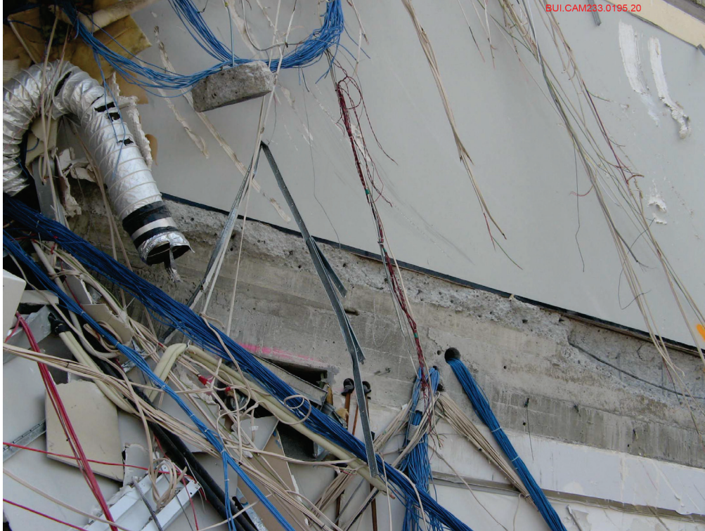
Figure 8-12 Photo of fractured slab reinforcement at slab-wall interface (Jury and Sharpe, 2011).
