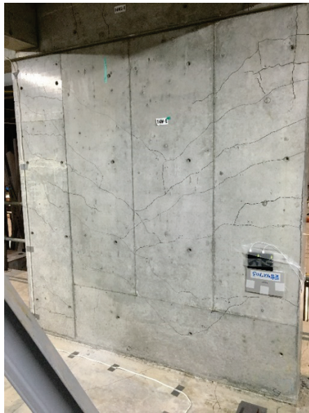
(a) Wall damage at 1st Floor
