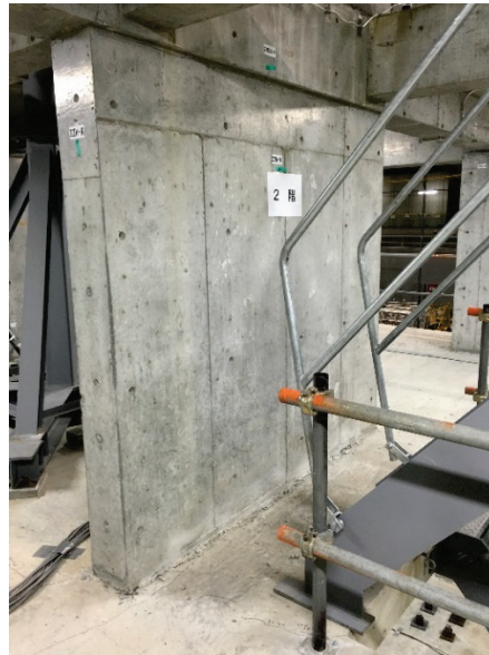
(b) Wall damage at 2nd Floor
