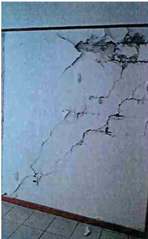
Figure 10-20 Damage to interior masonry walls in apartment unit (Dirac Ingenieros Consultores, 2019b).
